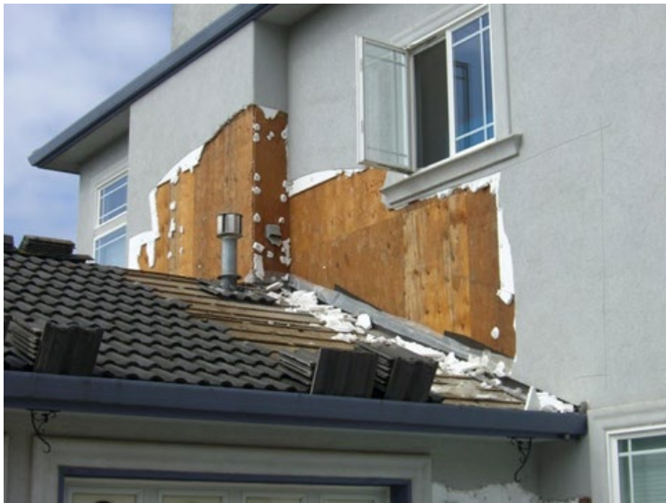
Residential Water/Mold Damage
